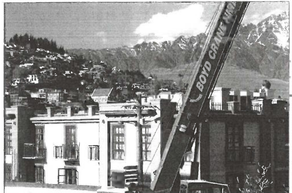
Man Street again: the giant Perron/Sofitel development, a source of bitter dispute with local residents about the height above the street.
